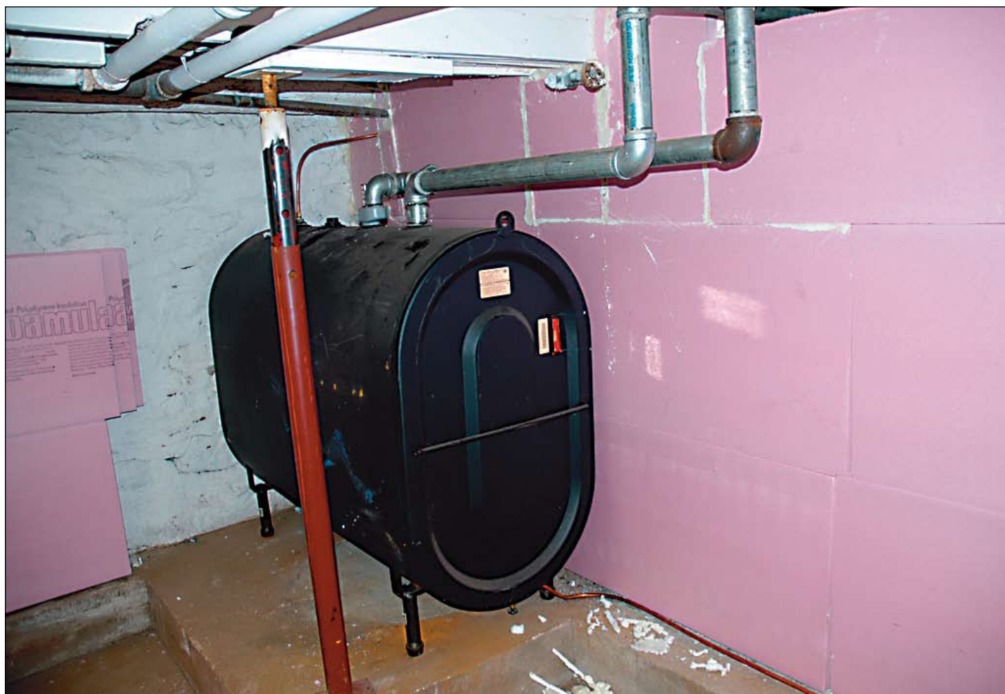
This fuel oil tank's days are numbered, thanks to a geothermal system being installed in Claudia Barritt's basement. Note the pink insulation being applied to the walls, which will make her home a "thermal envelope."
