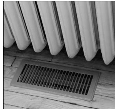
The old and the new energy conveyance systems in Paul Auerbach's home. The warm or cool air now comes through the vent in the floor. Auerbach will have the radiator removed once the price of scrap metal comes back up.
